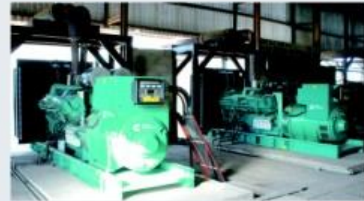
Cummings Diesel Generators
